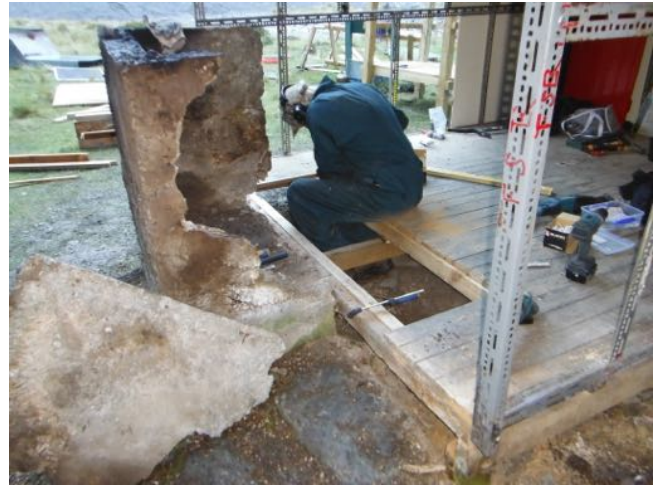
New joists and floorboards. Note broken Fireplace
