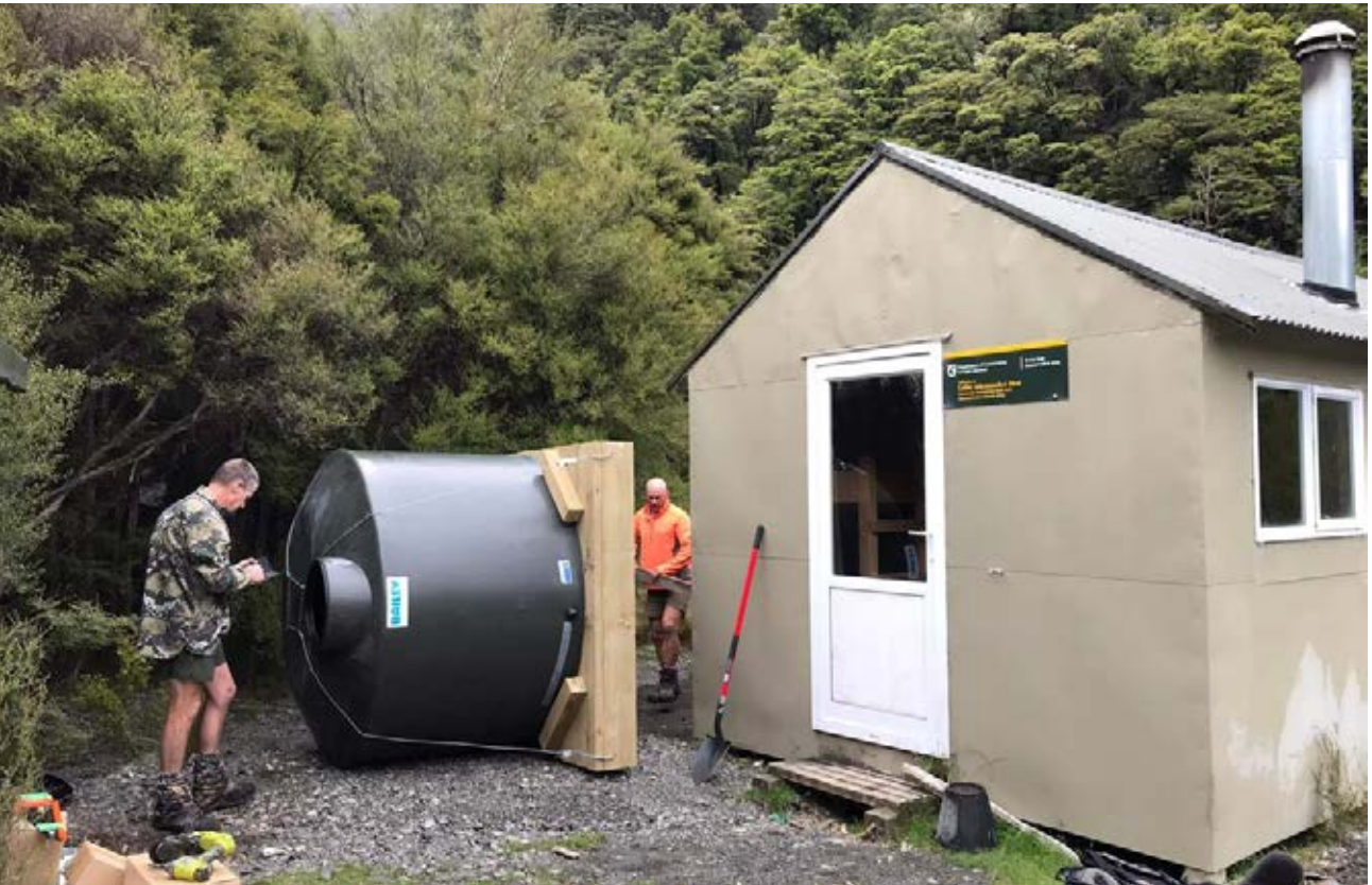
NZDA Marlborough and DOC installing a new water tank at Lake Alexander Hut
