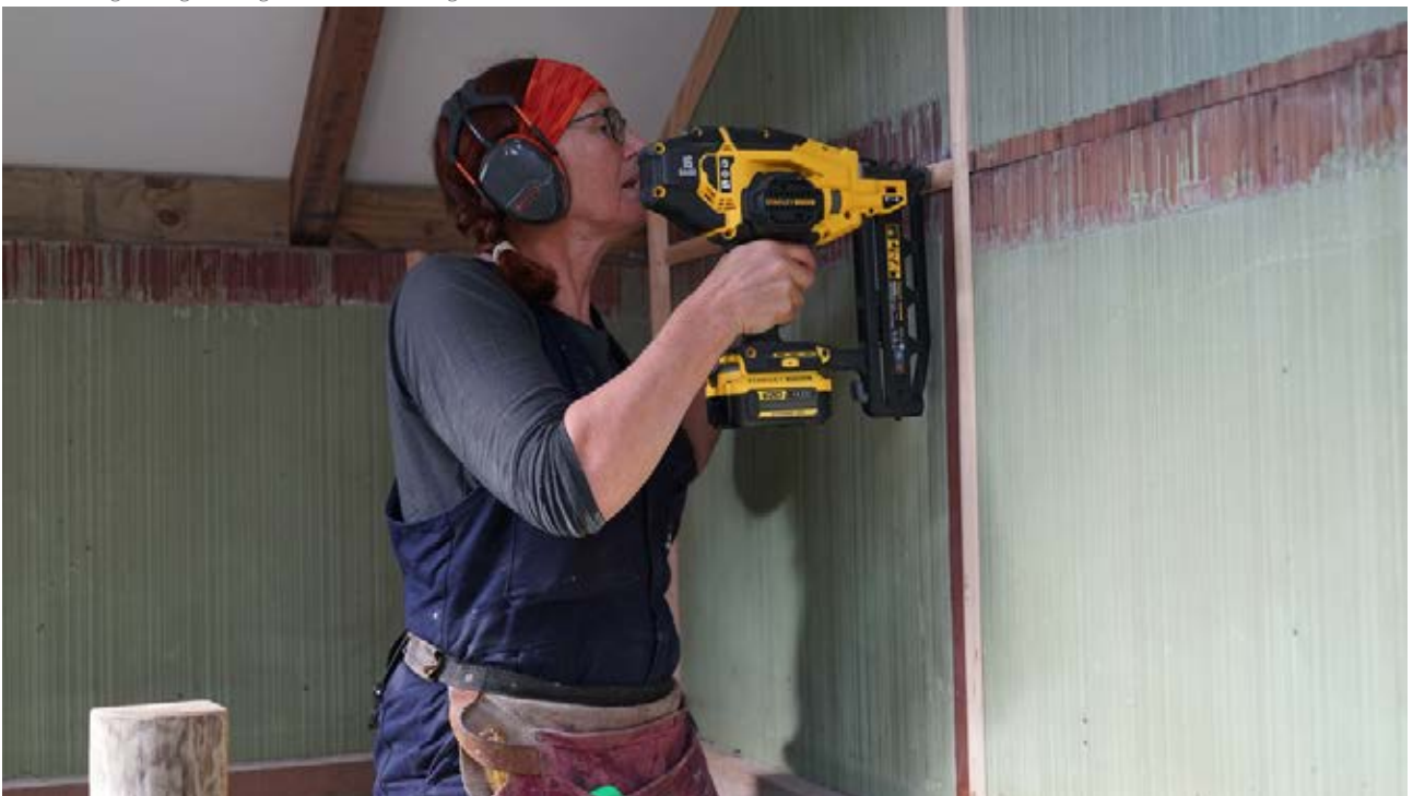
Fiona Burleigh fitting beading to the internal lining at Diane's Hut, Ruahine Forest Park
